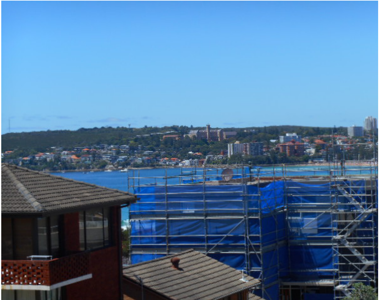
View affected from Balcony (standing) at Unit 5/55 Queenscliff Parade (Level 1)
